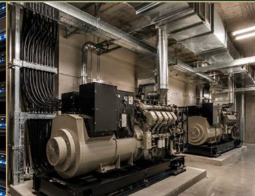
Backup Power (Generator)
