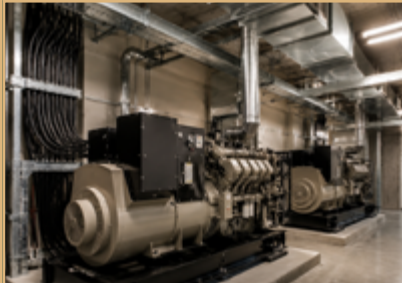
Backup Power (Generator)
