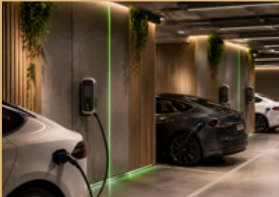
EV Charging Points
